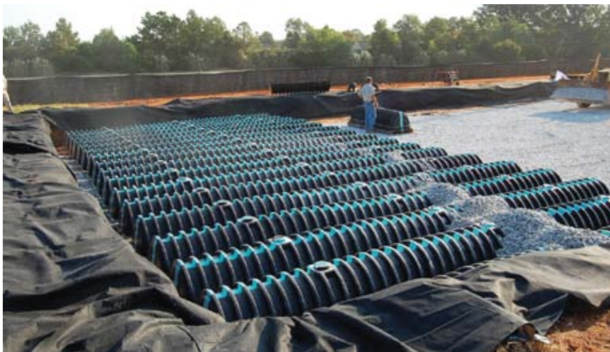
Choosing to detain storm water underground saved the owner 22,000 sq ft and about $166,000.
