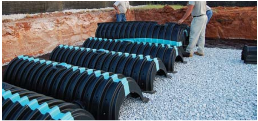
The site’s approximately 460 chamber units provide more than 21,000 cu ft of storage.
