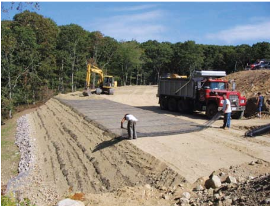
The housing developer on this mechanically stabilized earth job in Westerly, R.I., was able to develop additional lots on the property by using the structural solutions.
