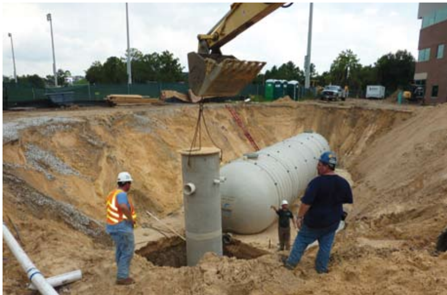
The system required a tank large enough to accommodate seasonal heavy rainfall.
