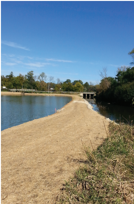
The project was designed to prevent future damage to the slopes while still allowing access to the outcropping stone fishing piers.
