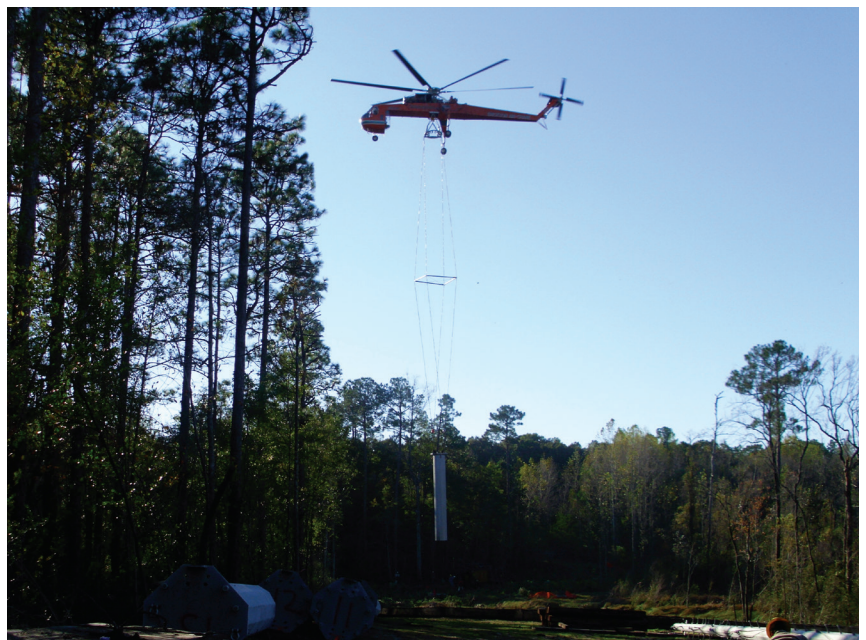
To avoid disrupting the sensitive wetlands, helicopters were used to carry in materials, install a portion of the line and haul away debris.
