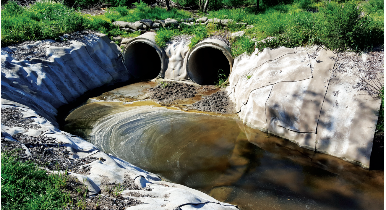
After the carrying capacity of the double-barreled culvert system was restored, GCCM was applied to prevent erosion of the exposed, non-vegetated bank at its output.
