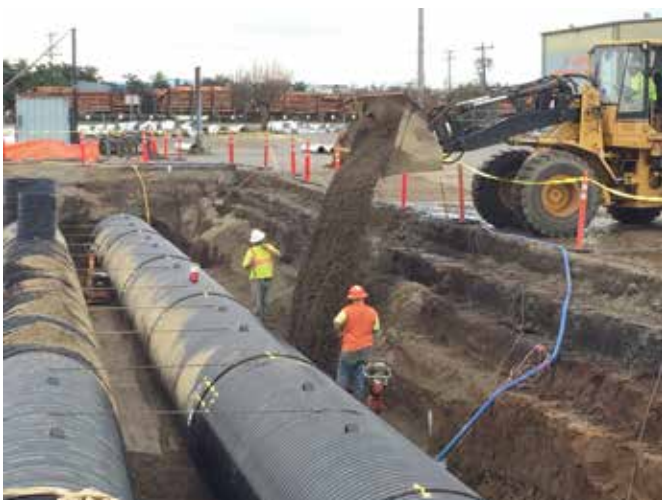
Crushed rock backfill was compacted in layers, allowing the corrugated steel pipe to support heavy-duty forklift traffic.
