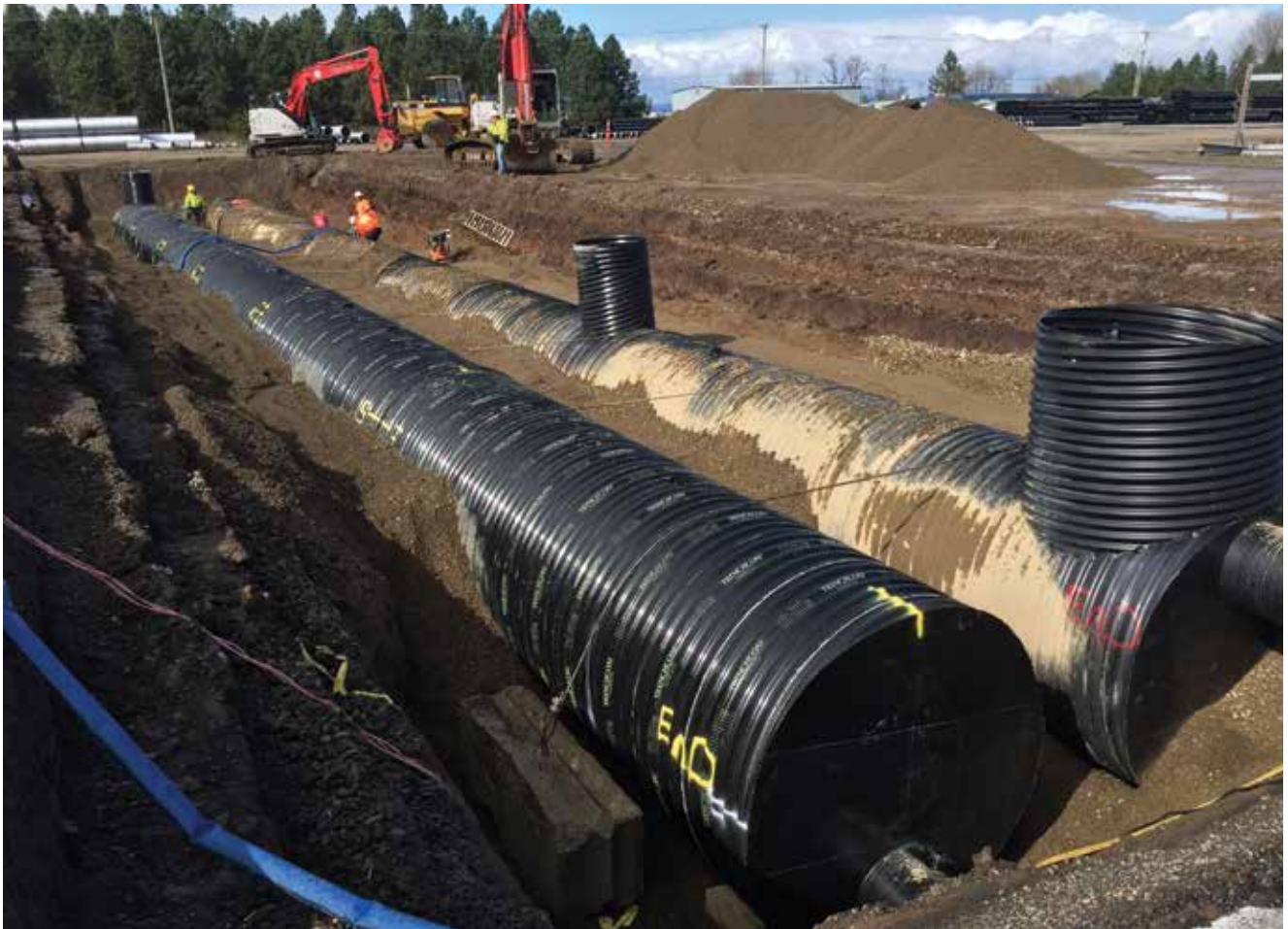
The storm water detention system consists of two 140-ft runs of 78-in.-diameter corrugated steel pipe.
