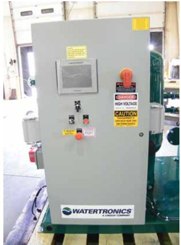
The pump station's programmable logic controller outputs data about the building's non-potable water supply.
