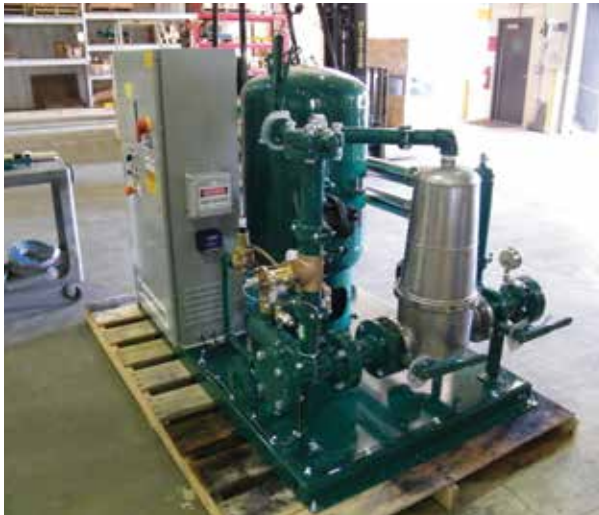
The submersible pump provides the complete flow and pressure required to operate all non-potable fixtures in the building.
