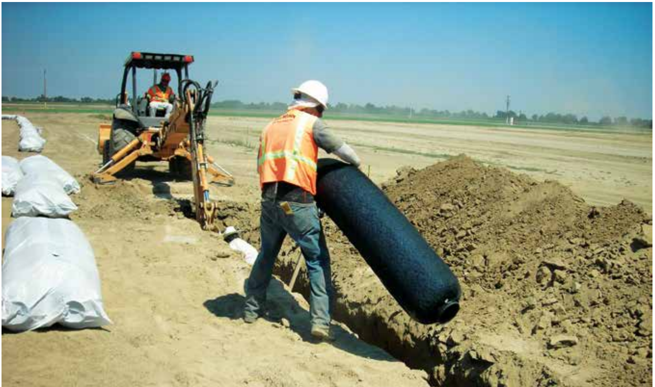
The underground drainage system at a Denver mixed-use development helps remove storm water from the foundation of the buildings.
