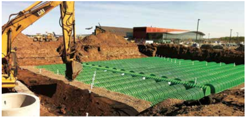
The underground chambers at Duluth International Airport allowed designers to work around challenging terrain and existing infrastructure.
