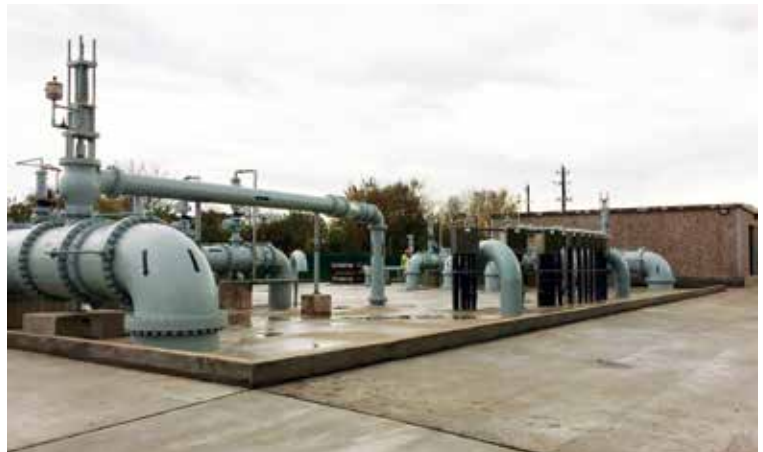
During dry weather, the station alternates the pumps to evenly distribute wear.
