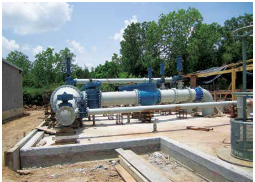
The new lift station has a current capacity of 33.12 mgd and an ultimate capacity of 42 mgd.
