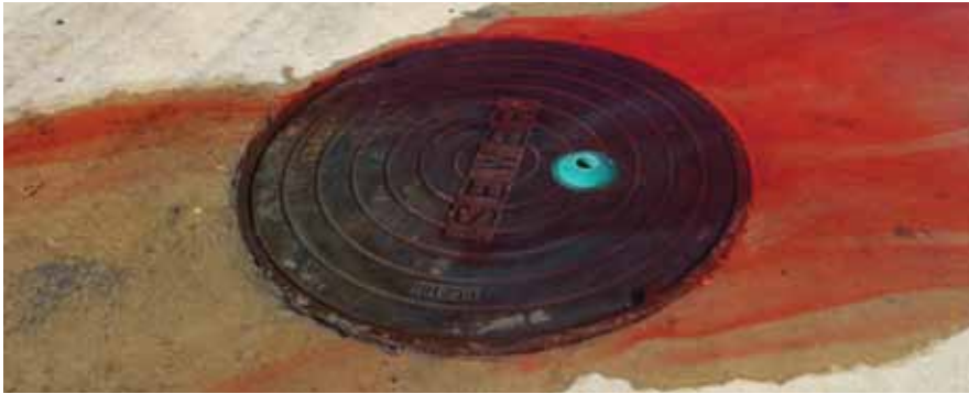
The venting device diverts most storm water during rainstorms and vents the system of corrosive gases during dry weather.
