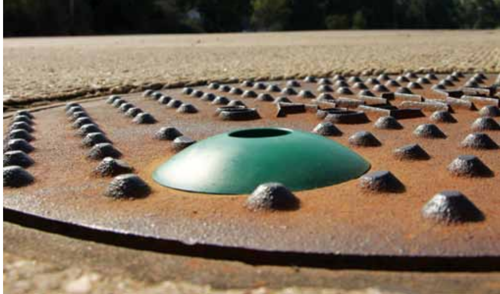
The device creates a raised vent hole that is \frac{5}{8} in. higher than the manhole cover.
