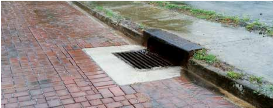
Permeable pavers at work during a rain event.
