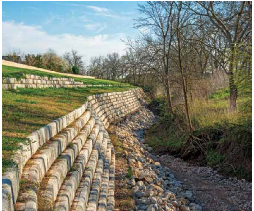
The solution includes a gravity retaining wall system coupled with a dual-level subsurface sheet piling wall for soil stabilization.
