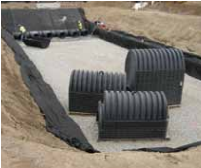
Engineers designed a storm water management system that contributed to the sustainability of the site and LEED certification standards.
