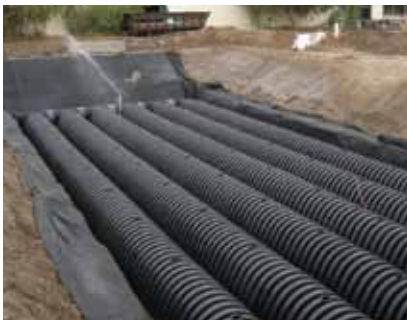
The chamber system allows the treated water to be detained and infiltrated into the groundwater aquifer below.
