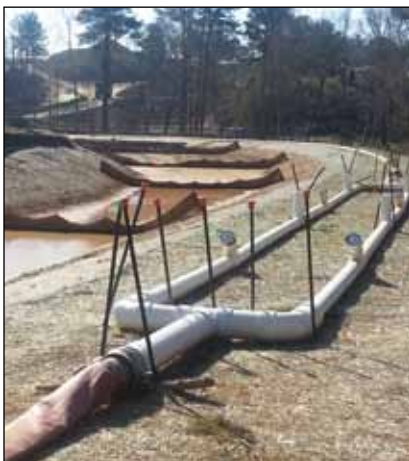
Top: A sediment pond with pump and treatment system. Bottom: A dual manifold system.
