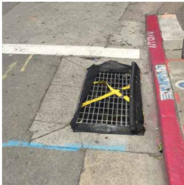
A correctly installed sediment control BMP (drain inlet filter) is shown here.
