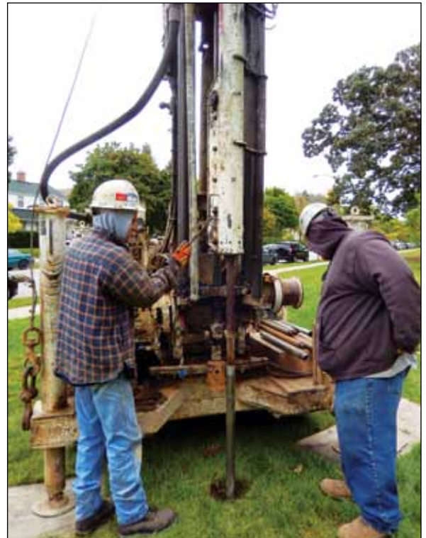
Workers perform subsurface exploration to confirm consistency of the control and managed test sites. Multiple 6-ft borings were drilled using an ATV-mounted drill rig.
