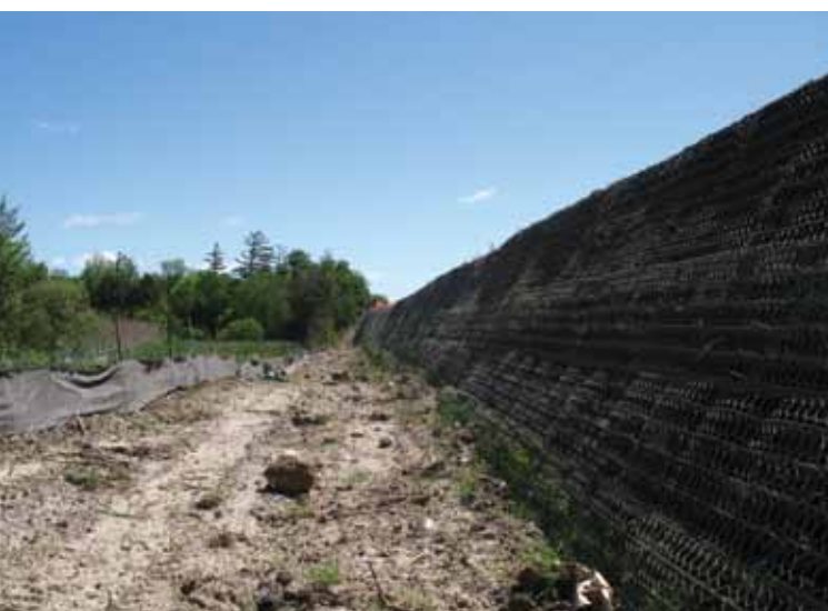
The wall used a prefabricated modular system made from hexagonal double-twisted wire mesh to reinforce the 60-degree slope.
