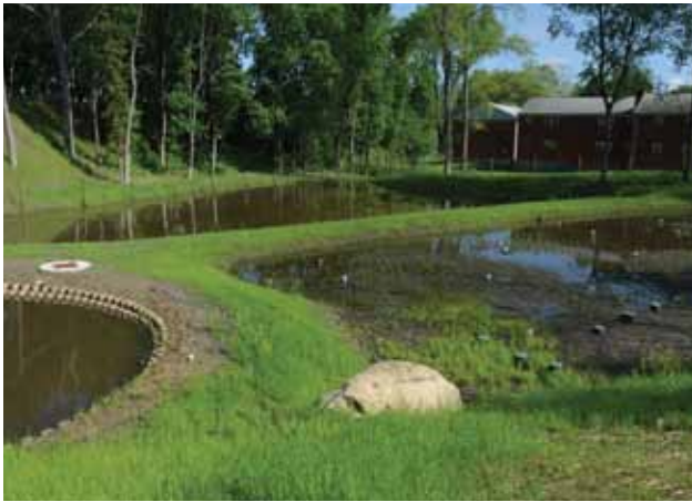
The subsurface flow gravel wetland traps and treats 85% to 95% of the sediment and suspended solids passing through it. Below: The completed wetland system
