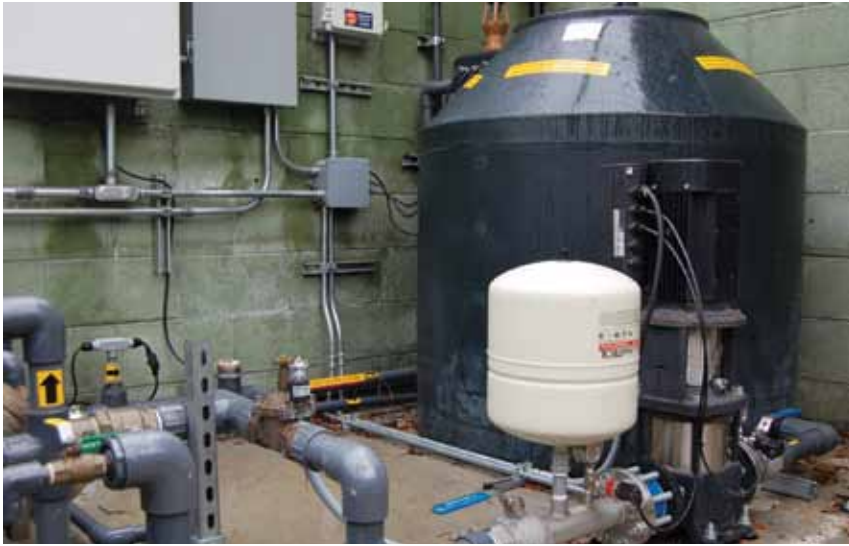
The tank and pump move treated water into the library for patron use.
