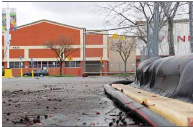
Working in small sections, installers connected the interlocking sections and secured the wattle to the asphalt by folding the tail and anchoring it into place.
