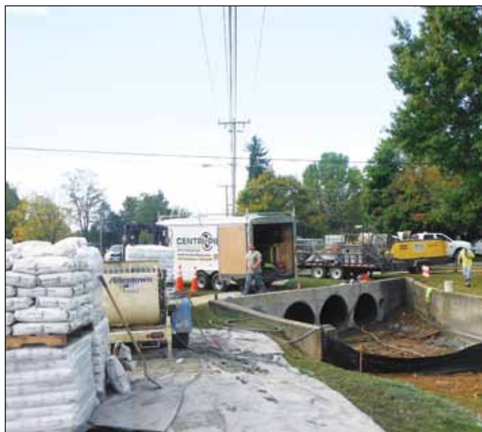
The culverts that required repair ran under one of the main thoroughfares in the town, making it less than ideal to close the street completely during the work.
