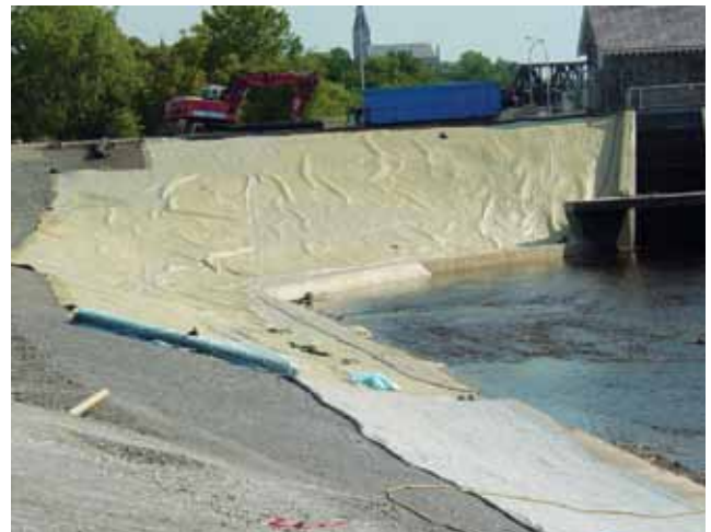
As the hydropower facility was being constructed, a leak in the dam embankment was discovered.
