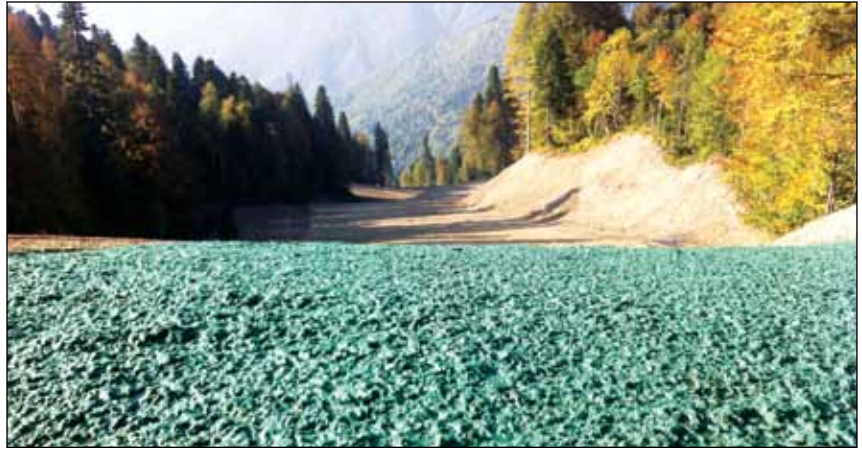
The altitude of the mountain range and vast distances of the steep slopes meant a lot of hose work, often with a harness for the applicator to ensure safety.
