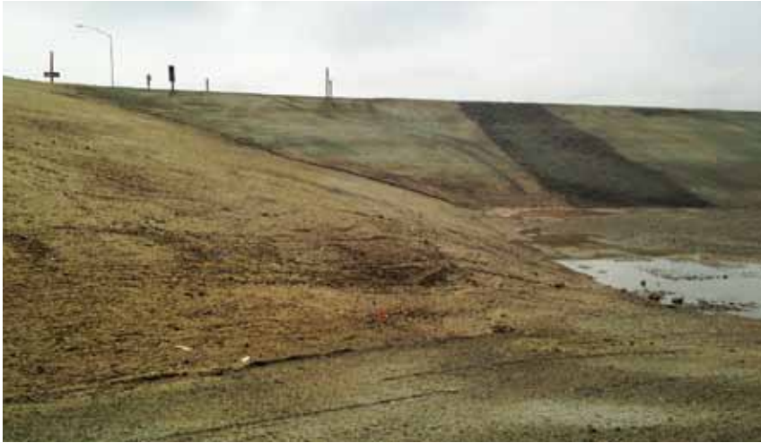
The test site after heavy rains
