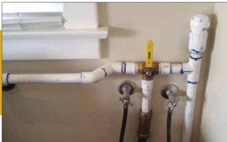
The Natural Resources Defense Council greywater system in Santa Monica, Calif.
