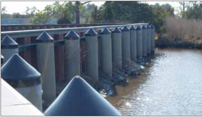
The floodwall held back rising waters from Hurricane Irene in August 2011, and damage from the hurricane was minimal.
