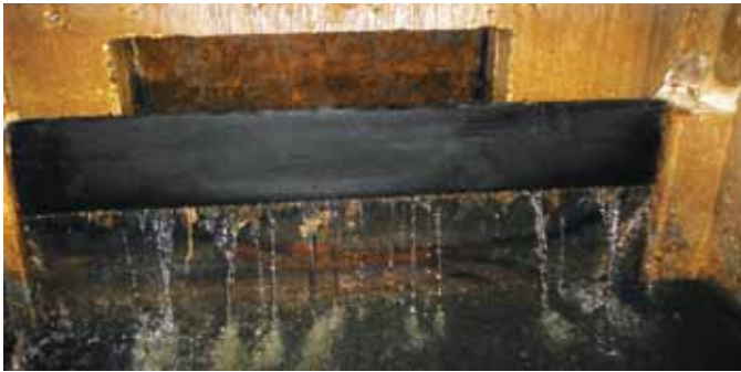
A monitored CSO control structure with backflow from the receiving stream infiltrating through the weir board
