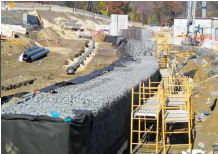
The gabion wall portion of the Croton Water Treatment Plant project began in 2012.
