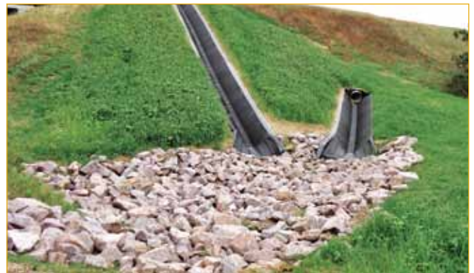
A channel-lining system was installed after the riprap failed multiple times.
