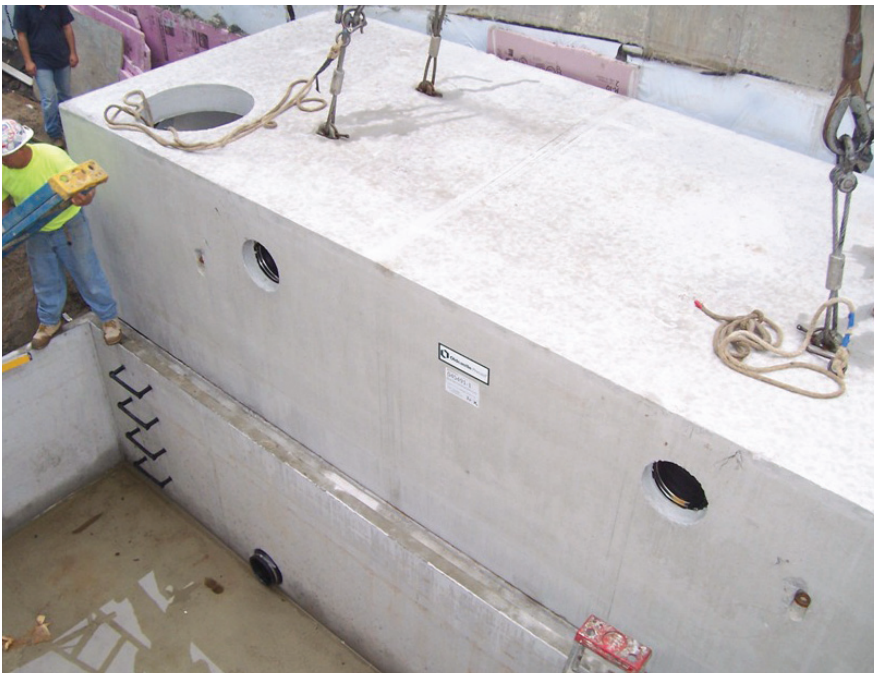
The storm water harvesting system will reduce potable water demand as well as runoff into the combined sewer system.
