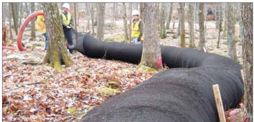
The Hemlock Farms community in Pennsylvania’s Pocono Mountains is a 4,600-acre development that contained 3,600 homes, 75 miles of roadway, 100 acres of lakes—and no modern storm water management.
