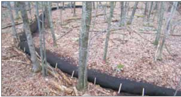
The solution was designed to blend into the landscape and treat runoff along the entire flow path.
