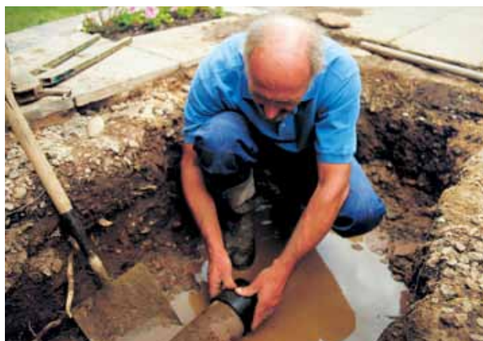
An exterior water line overflow is one sign of an I&I problem.
