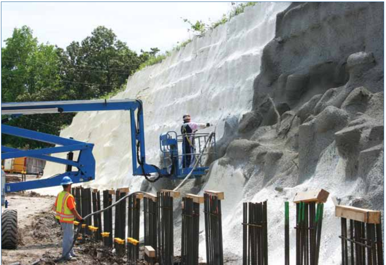
The shotcrete wall was 25 ft high and required the use of an aerial lift to spray the upper portions from a man basket.
