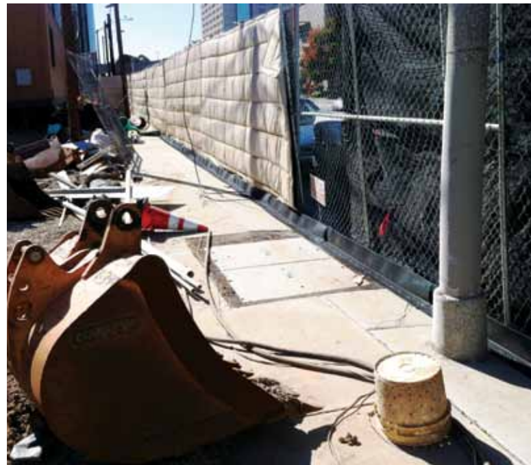
The storm water pollution prevention plan is aided by a perimeter storm water BMP designed to seal to hard surfaces.
