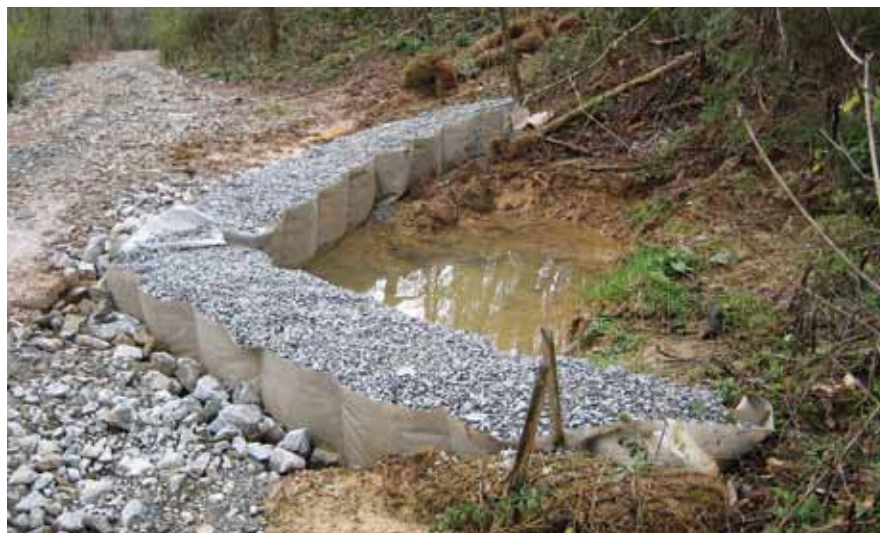
Runoff from a highway construction project in Tazewell, Tenn.
