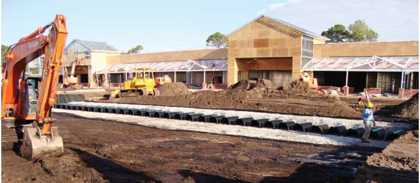
An underground chamber system solved the site's land-constraint issues and was designed to function as a detention solution with no infiltration. (Photo courtesy of Tanger.)
