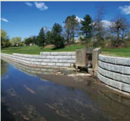
The engineer designed the channel walls to meet the creek's 100-year flood levels.
