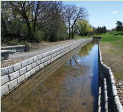
The design of the channel allowed the existing bridges to remain intact.
