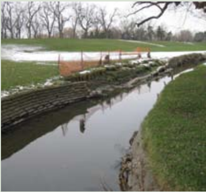
The Two Mile Creek channel originally was armored using bags of cement that hardened into walls.
