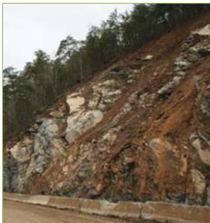
A major rockslide in Tennessee threatened Highway 64 and the Ocoee River.
