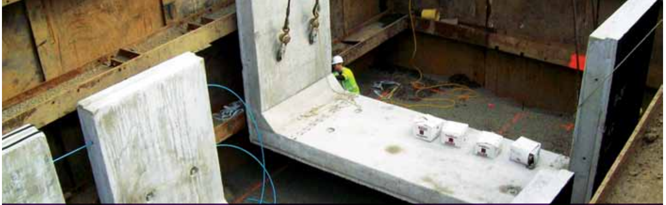
In New York City, 23 precast concrete sections were installed to create the Bronx River CSO Netting Facility. Photo courtesy of Garden State Precast.
