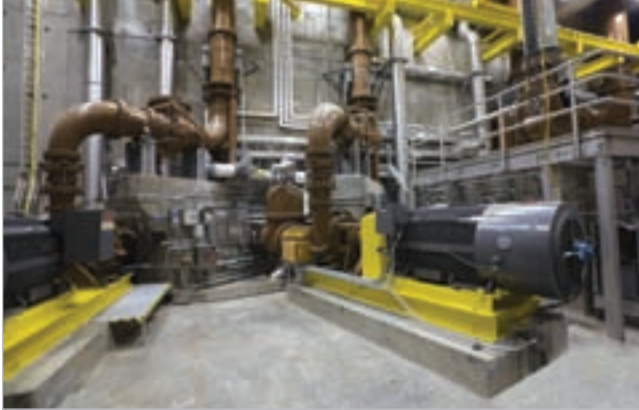
The Swan Island Pump Station serves the West Side CSO Tunnel; it will also serve the East Side CSO Tunnel once that project is complete.
