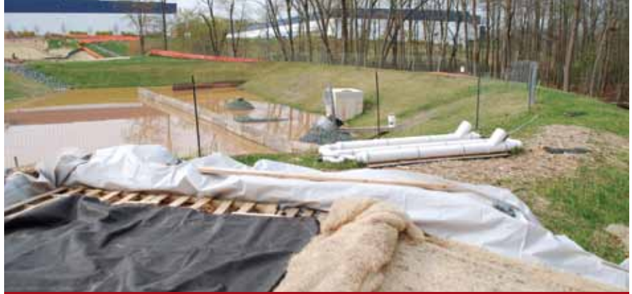
A dirt bag, shown here in front of a storm water basin, captured sediment.
