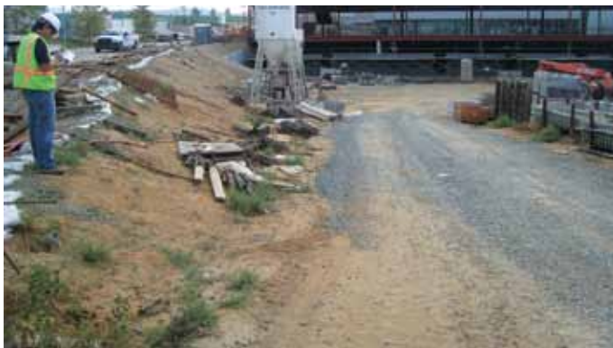
Construction general permits create an environment of potential conflicts of interest among involved parties when a typical contract setup is used.
