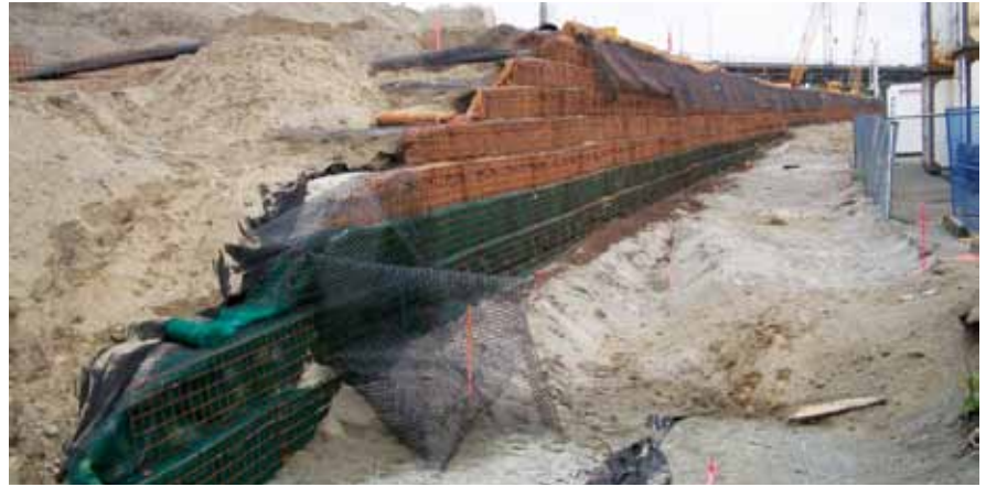
The slope design was estimated to be able to withstand a 975-year seismic occurrence.
