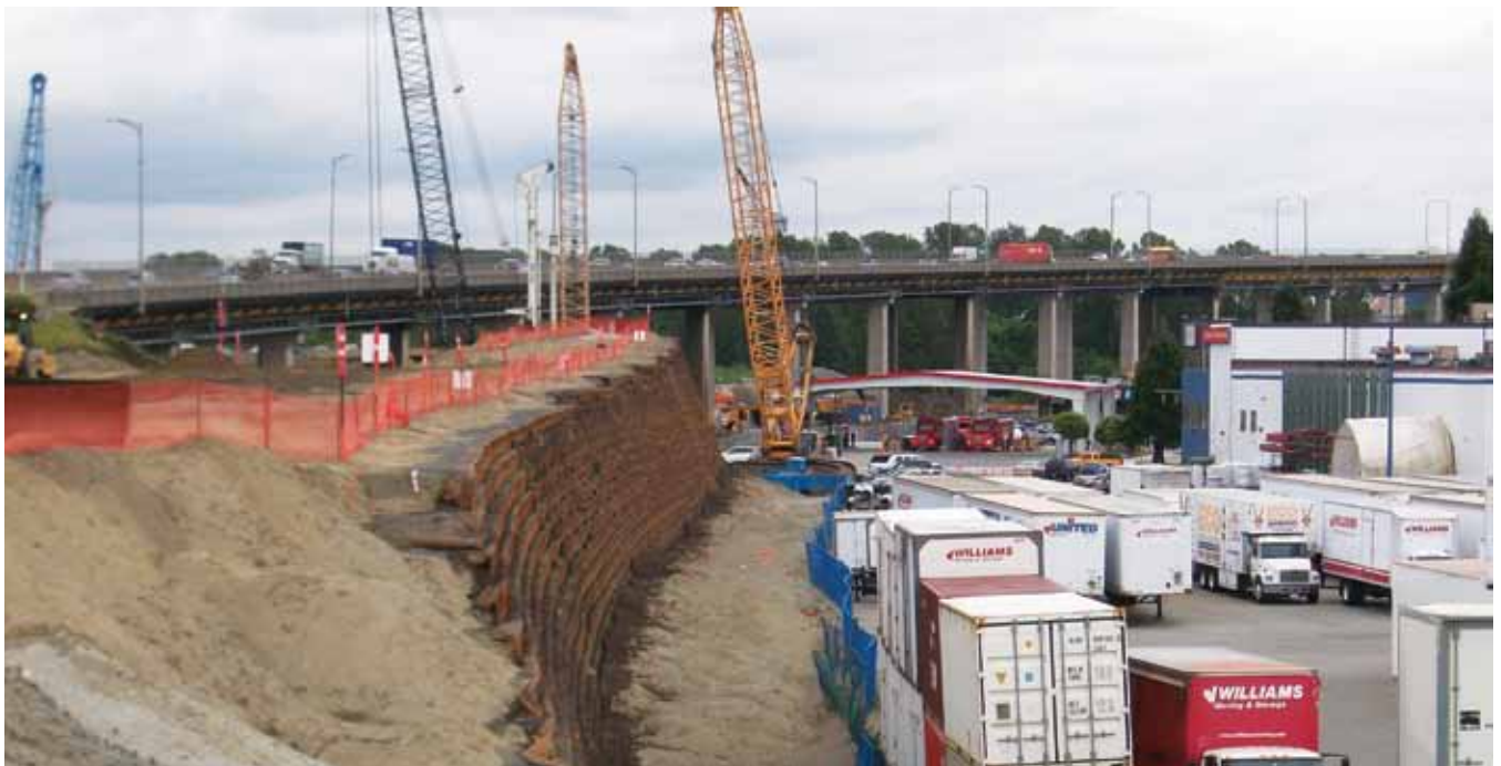
British Columbia's new bridge includes more than two dozen slope retention systems and two retaining wall installations.
