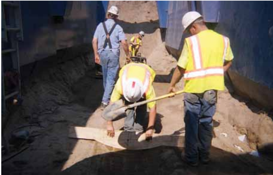
Workmen prepare to lay the pipe for the Sanitation District No. 1 installation.
