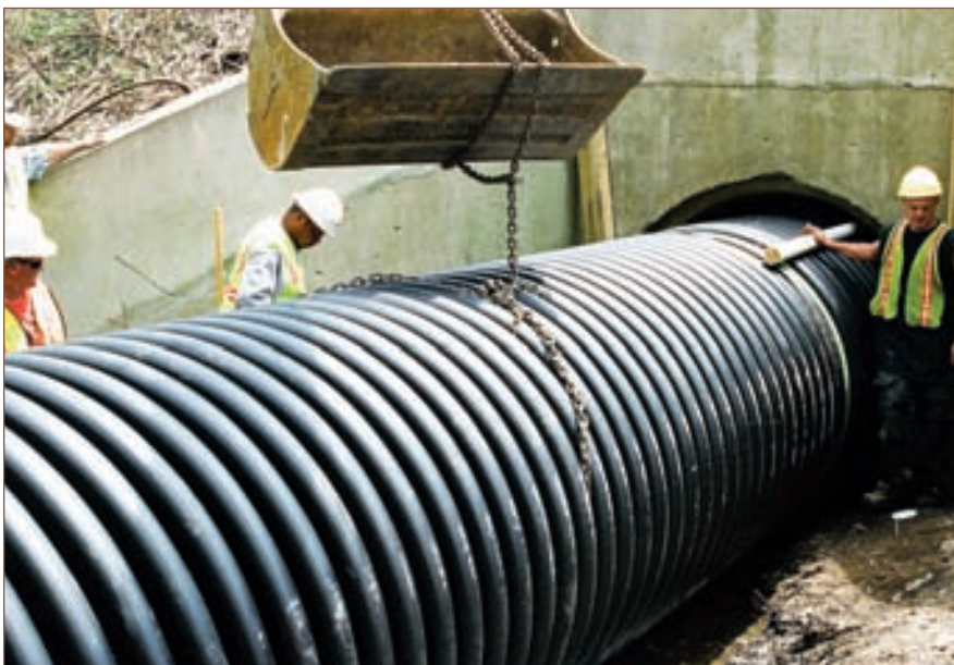
With the help of a backhoe, a four-man crew joined and slipped new pipe sections into place.
