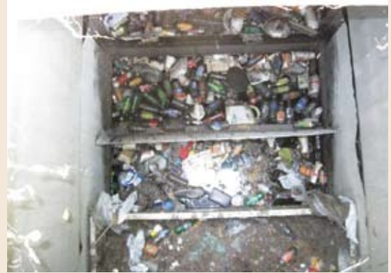
A device in a major retailer's parking lot that went uncleaned for four years.
