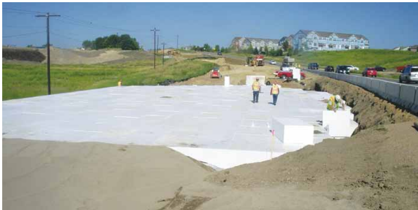
A combination of expanded clay lightweight aggregate and expanded polystyrene blocks provided a way to manage storm water runoff and was an alternative to building a bridge.
