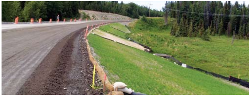
Live water and perimeter control, slope stabilization and drainage contours are important considerations on active sites.
