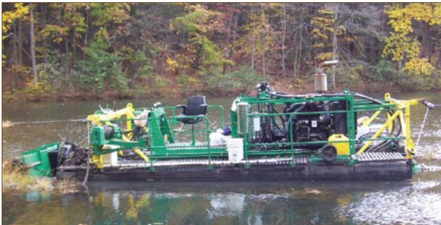
Using pumps and filter bags, workers hydraulically dredged approximately 7,000 cu yd of material from the bottom of Lake Henrietta.
